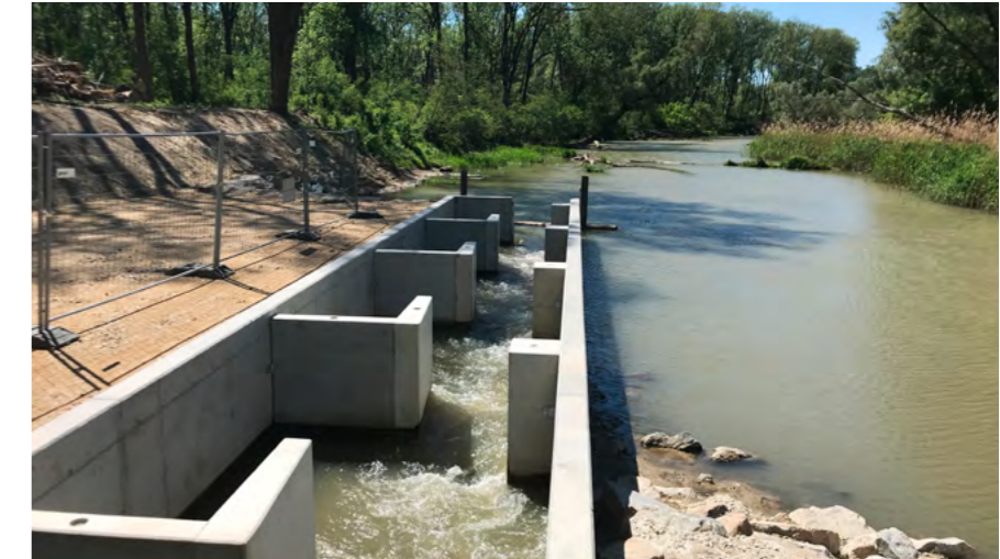
Barrier-free fish passage through new vertical slot facilities in the Greifenstein "Gießgang"
