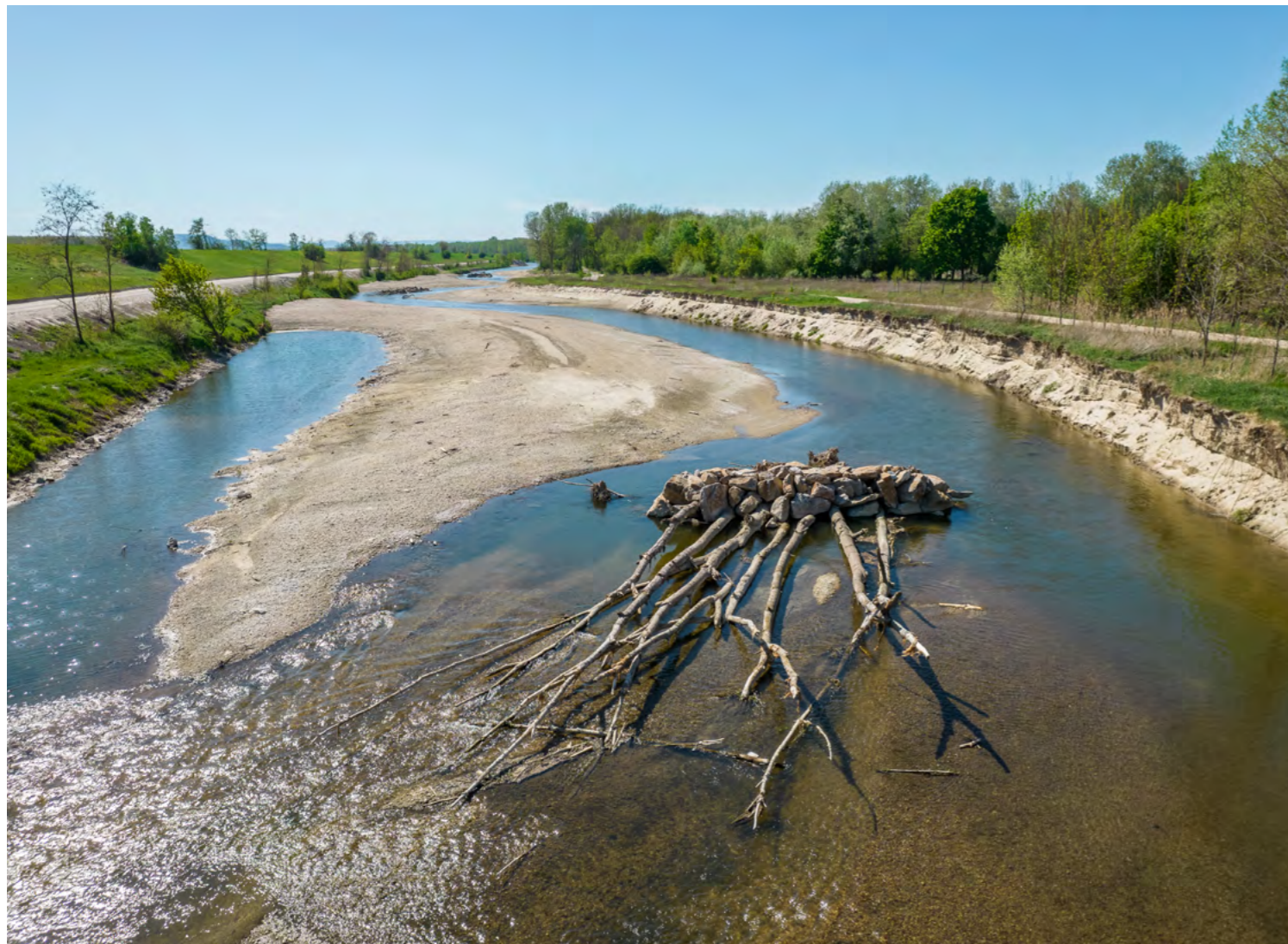
Altenwörth dynamic bypass river: about 30 hectares of new river habitat have been created in the LIFE Network Danube Plus project.
